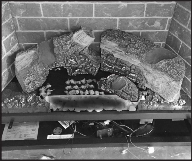
Figure 6. Burner Log Installed
