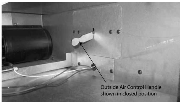
Figure 3.20 Outside Air Handle Shown on Right Side
