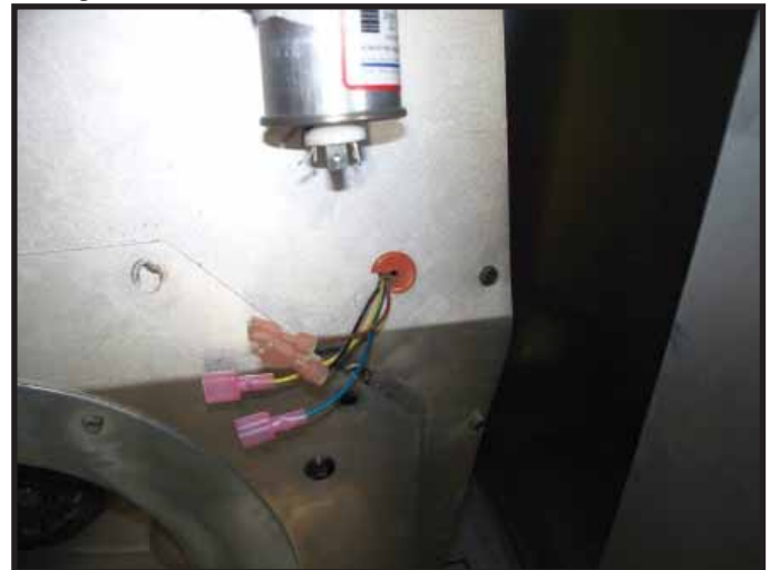
Figure 3.7. Grommet and Wires
