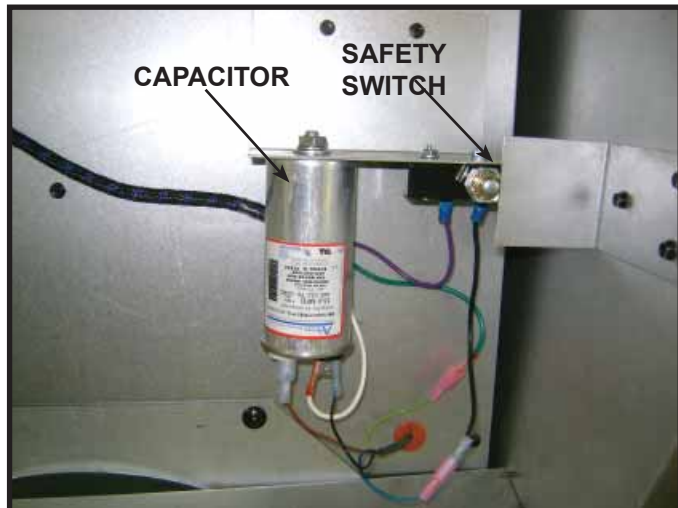
Figure 3.5. Capacitor and Safety Switch
