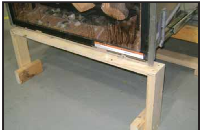
Figure 1.5. Appliance Resting on Field-Constructed Support
