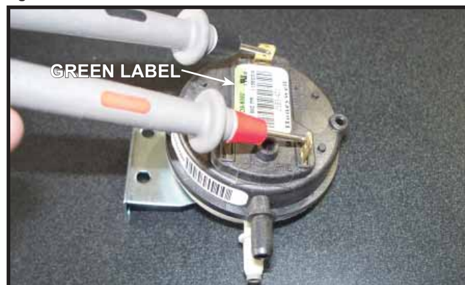
Figure 3.2. Test Intake Pressure Switch
