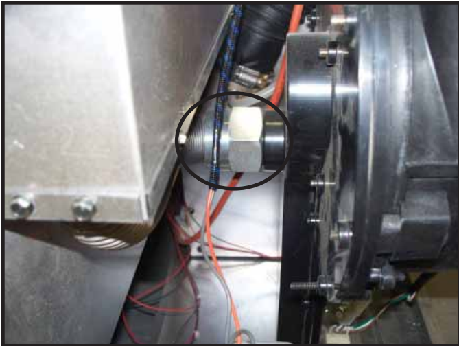
Figure 3.16. Disconnect Heat Exchanger
