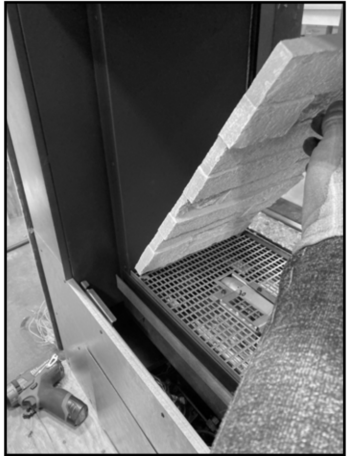
Figure 15 Position Side Refractory Panel
