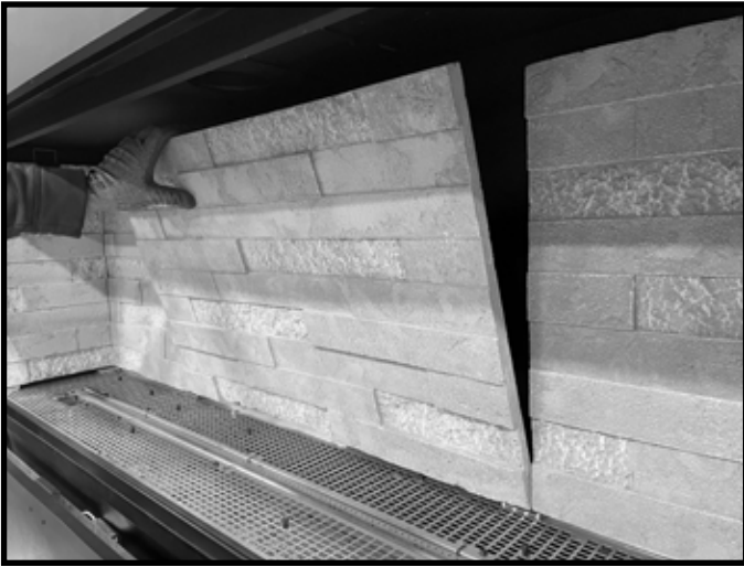
Figure 33 Position Center Back Refractory Panel
