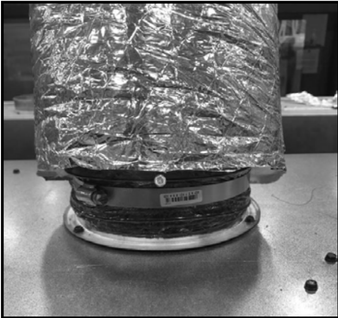
Figure 4 Flex Vent Properly Installed
