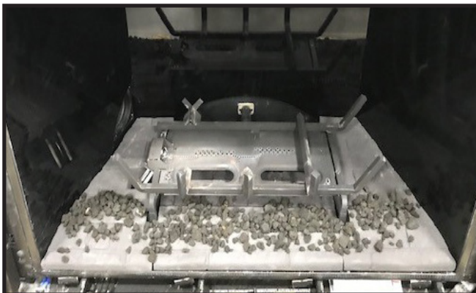
Figure 3 Logs removed from appliance
