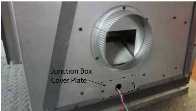
Figure 4.1 Junction Box Cover Plate
