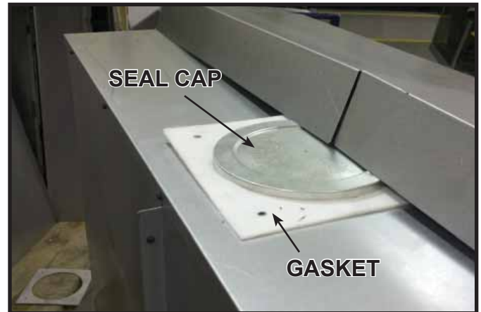
Figure 9.2 Seal Cap and Gasket Location
