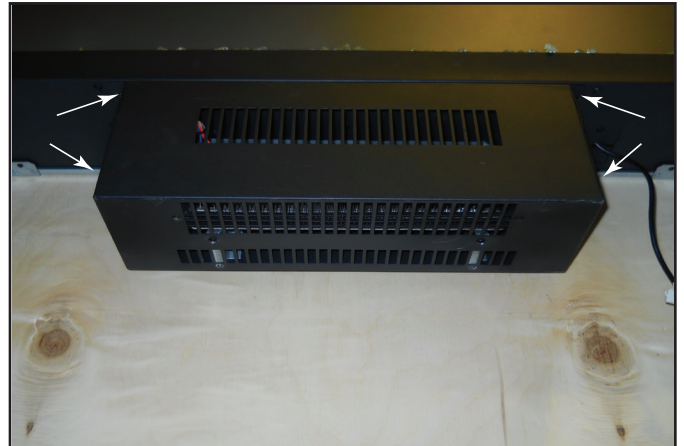
Figure 14 Fan Box Fasteners
