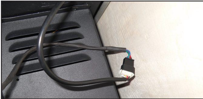
Figure 12 Lighting LED Connection
