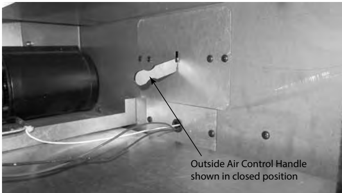
Figure 3.20 Outside Air Handle Shown on Right Side
