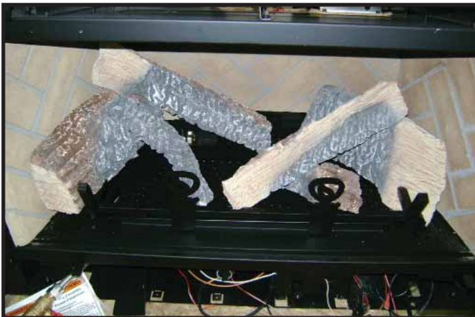
Figure 2. Refractory and Logs Installed
