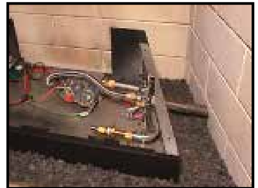
Figure 5 - Gas Line Connection
