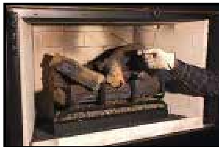
Figure 16 - Checking for Spillage
